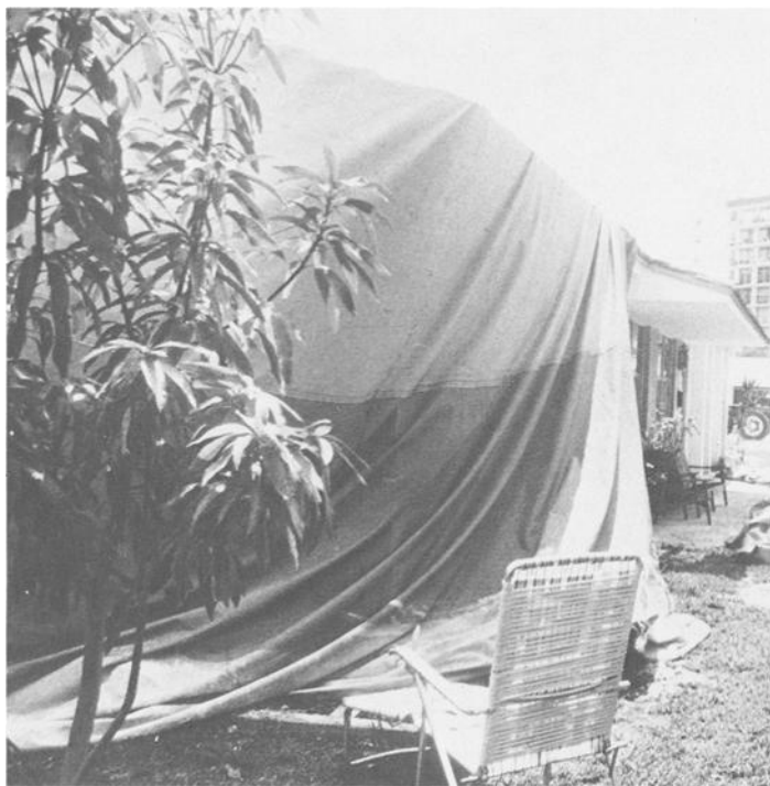
FIG. 1—A tent is assembled around the residence to create a nearly vapor tight enclosure.
